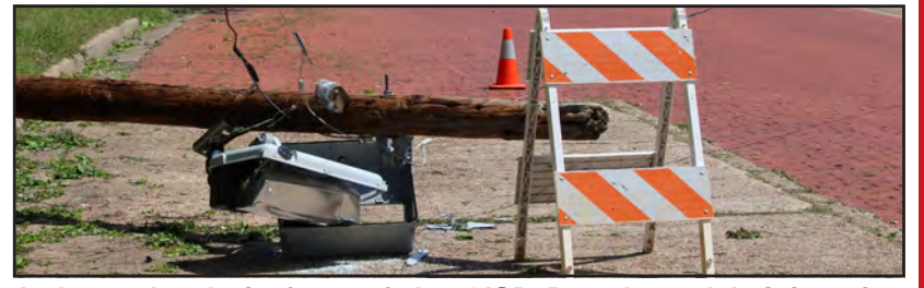
A downed pole in front of the GUSD Broadway Administration building was narrowed to one lane on Monday morning due to the low hanging wire. The damage was caused by Sunday's storm.
