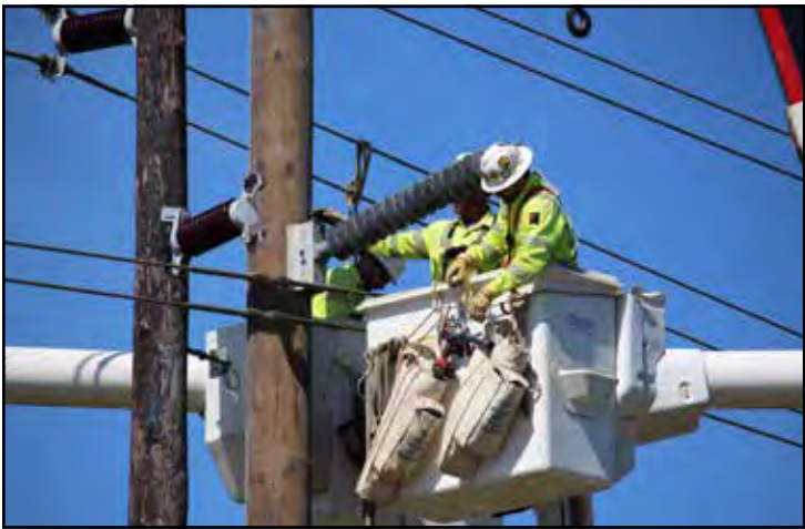
Linemen servicing equipment on Hwy. 271 North close to American Căanopy were almost a traffic stopper last week with drivers slowing down to watch the men replacing parts. Photo By Suzanne Bardwell
