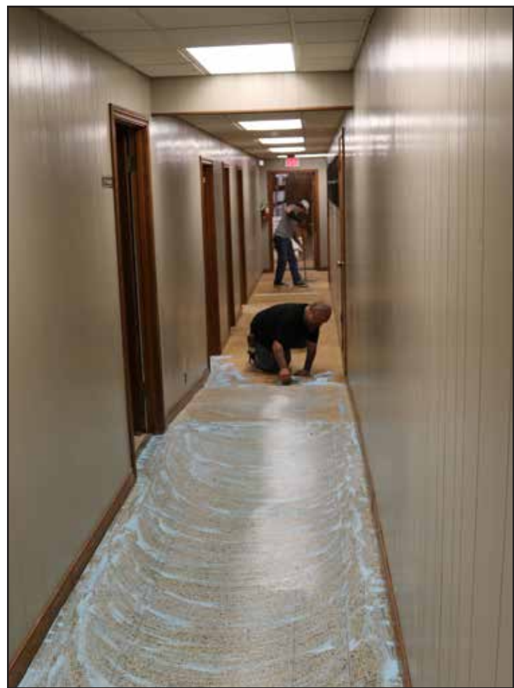
Workers prepare this hallway at City Hall for a new floor covering made possible by a generous donation by John Paul and Beverly Tallent.
