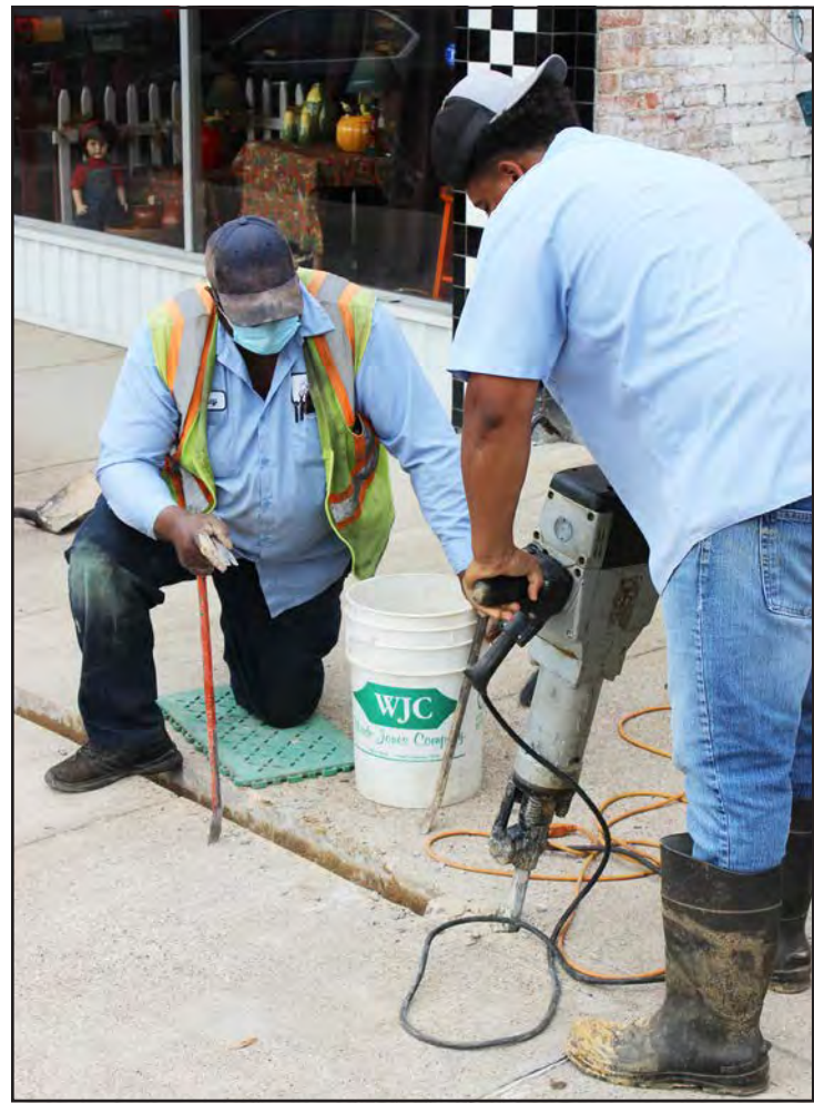
Gladewater public workers employees jack hammered concrete Monday morning to make way for conduit and electrical wiring for the downtown street lamps. Monday's work brings the downtown light project, funded by the Gladewater Economic Development Corporation, one step closer to being complete. GEDCO board member John Paul Tallent is overseeing the project.
