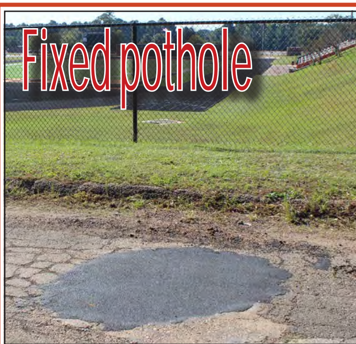
The last Pothole of the Week in front of Jack V. Murphy Stadium on Hendricks Street is no more. It is fixed along with the family of potholes that ran the length of the street to Gay Avenue. Kudos to city workers for the fix with hundreds of visitors coming to Gladewater for Bear football games, soccer, cross country meets and more the ride is now a much smoother one.
