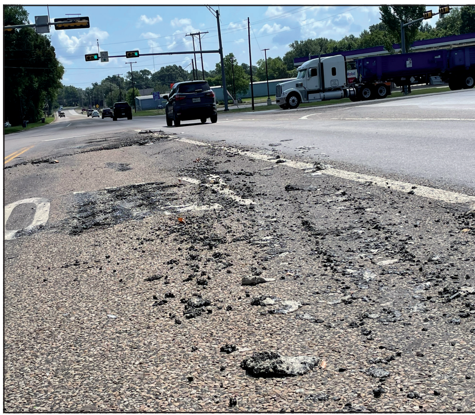
An as-yet-unidentified large vehicle caused thousands of dollars worth of damage to the roadway at the intersection of the loop and Hwy. 271 Monday morning. Evidently, a heavy vehicle's blown tire churned up the road surface and shredding markings as it was dragged across the surface. City of Gladewater personnel reached out to alert Texas Department of Transportation of the damage and develop an estimate for repairs.
