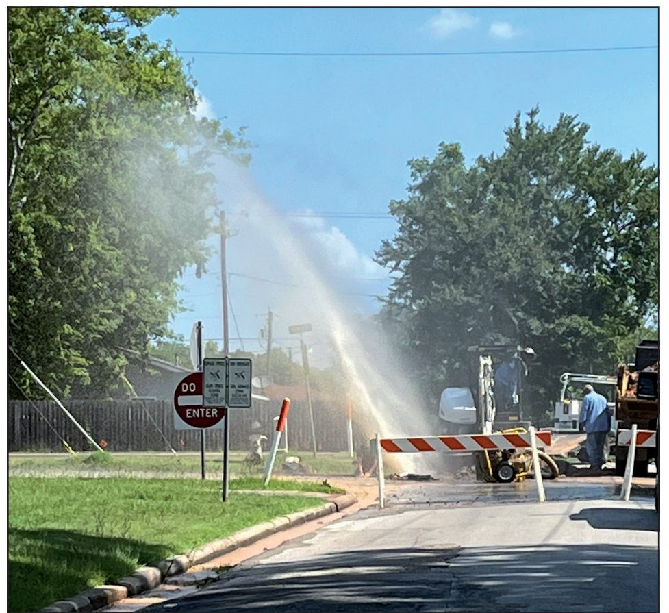
Water erupts from a line break at Saunders and Anderson Lane July 1 following a rupture in a two-inch line.
