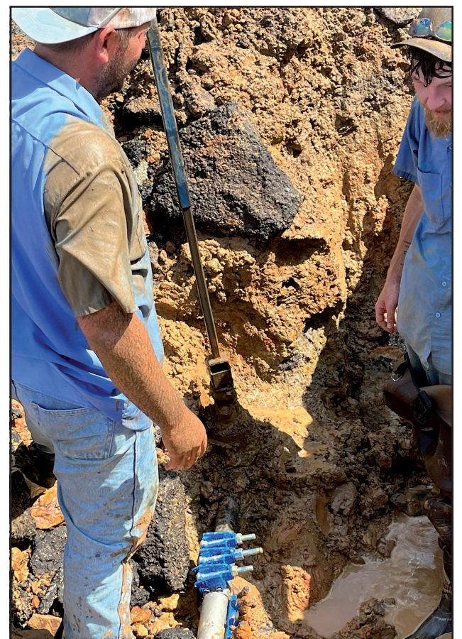
Gladewater Public Works crew members Seth Filkins (right) and Billy Williams stand in a three-foot hole next to a broken two-inch line at Saunders and Anderson Lane July 1. Repairs would have been easier, Gladewater City Manager Charlie Smith said, had personnel known the location of the valve buried next to the pipe.
